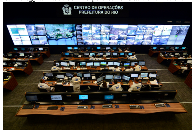
The Control Centre in Rio de Janeiro
